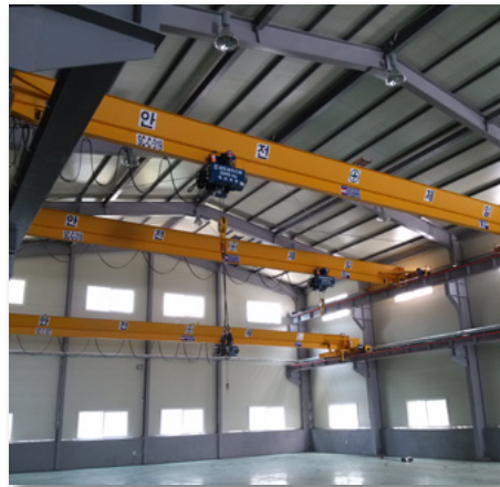
Single Overhead Hoist Crane
