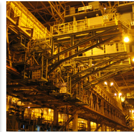
Wall Jib Hoist Crane
