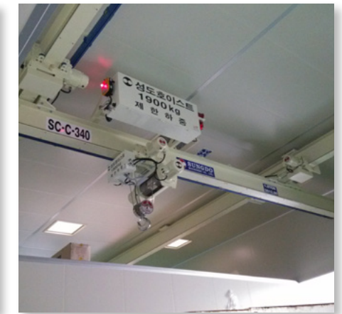
Clean Room Hoist Crane
